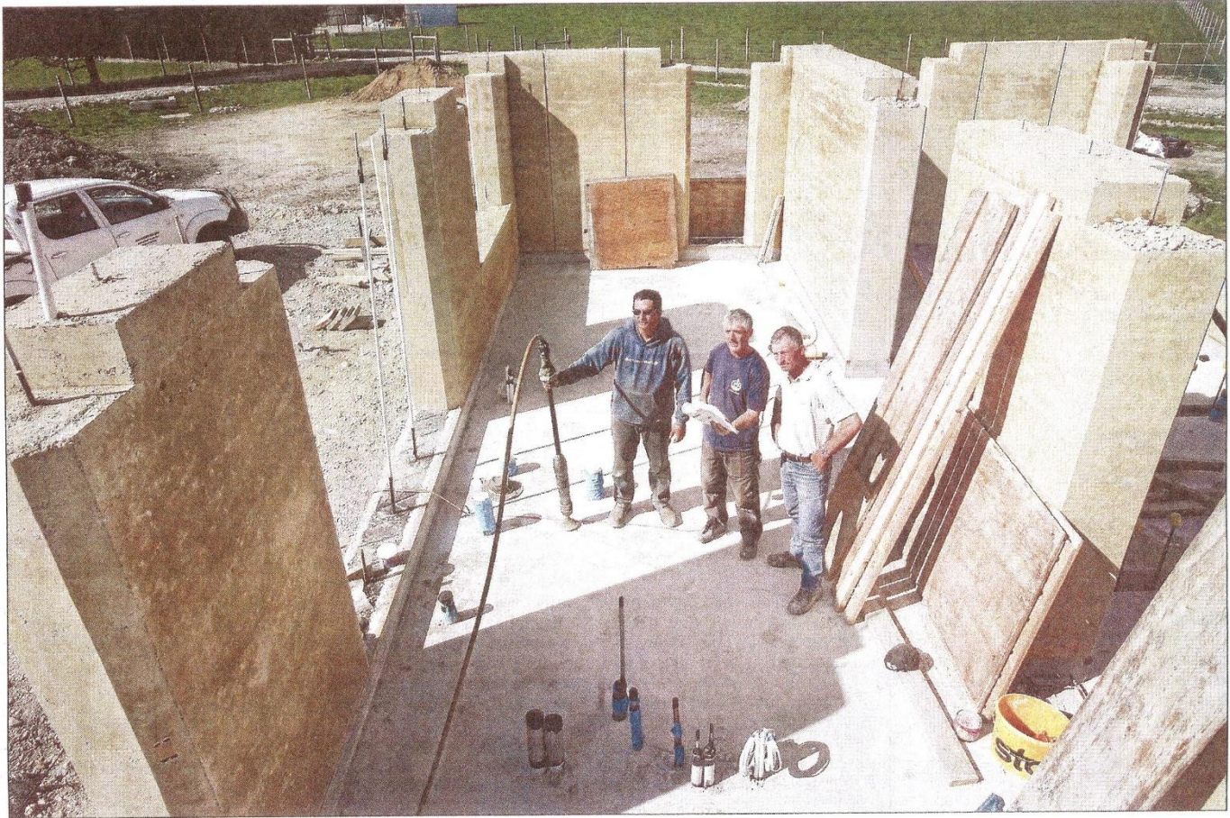
Earthworks: Standing in the Ruperts' rammed earth house near Peel Forest are, from left, Shane Edwards, Jimmy Cotter and Martin Rupert. Photo: JOHN BISSET/FAIRFAX NZ
